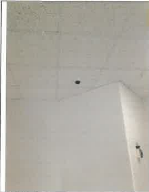
Exhibit A- Security cameras in hallway
